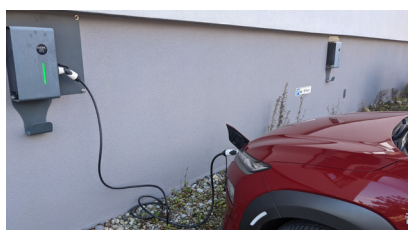
The electric charging station, which is fed by the photovoltaic system installed on our roof.
